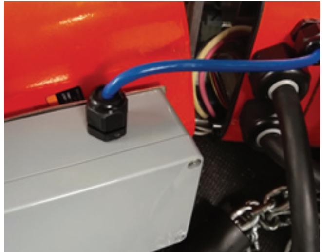
Figure 6: Cable Installed Between Both Glands
