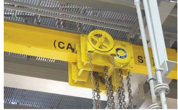
SPARK RESISTANT/EXPLOSION PROOF, 5-TON CHESTER ZEPHYR LOW-HEADROOM TROLLEY HOIST IN USE ON AN OFFSHORE OIL PLATFORM.
